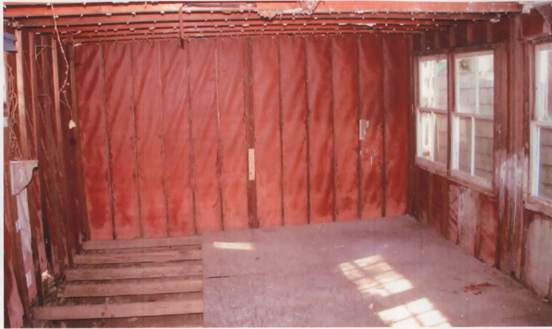
INTERIOR VIEW LOOKING TOWARD THE WEST WALL SHOWING THE PANEL FRAMING, WIGWARM PAPER LINING AND "SUNROOM WINDOWS" IN THE NORTH WALL. THE CEILING JOISTS WERE INSTALLED IN THE 1950S AND THE FLOOR JOISTS AND PLYWOOD FLOORING LATER.
