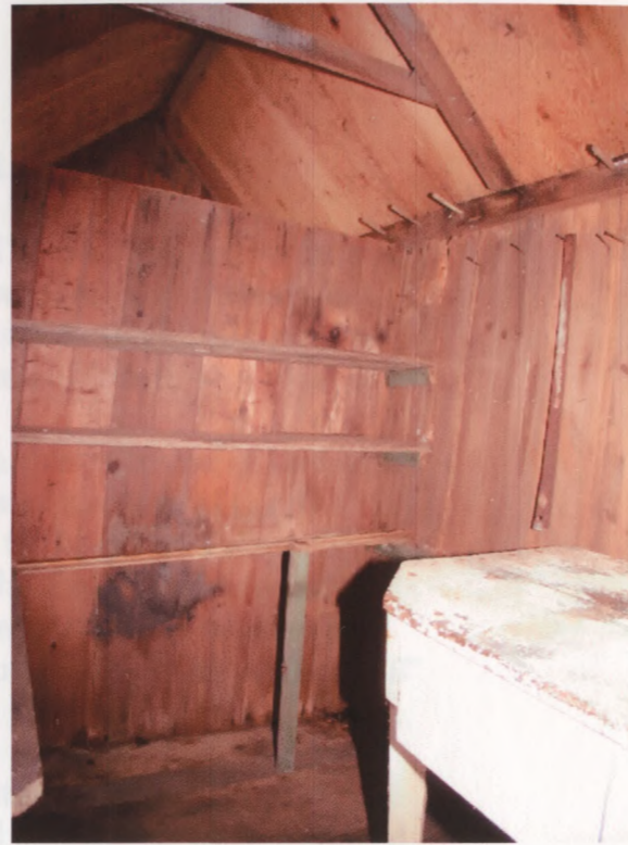
INTERIOR OF LARGER NORTH ROOM LOOKING SOUTH TOWARD THE DIVIDING PARTITION AND SHOWING THE PEGS SET IN THE PLATE
